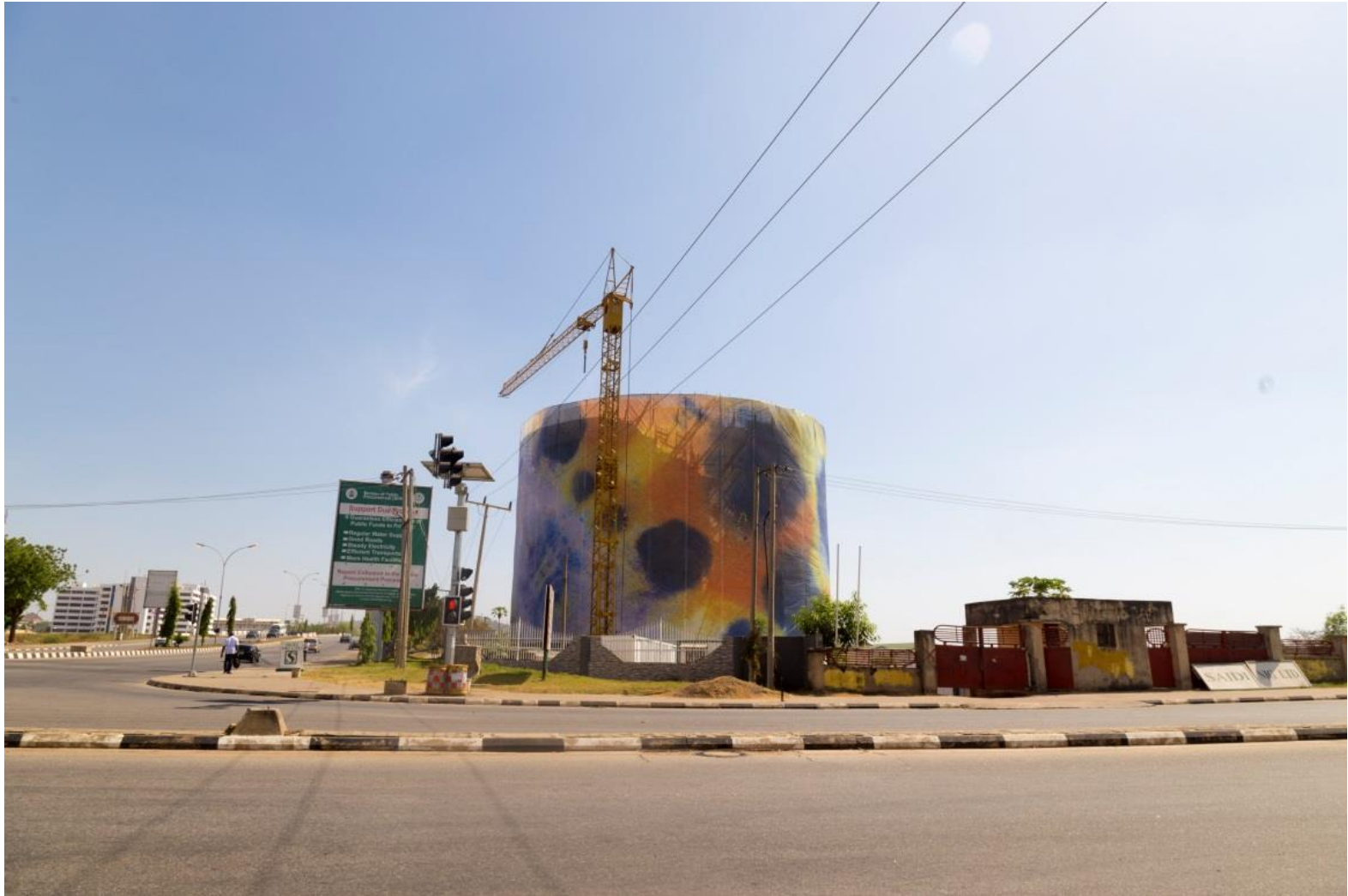
Public Art (Building Wrap of Ministry of Women Affairs & Social Development building as part of Go Woman Go!)
